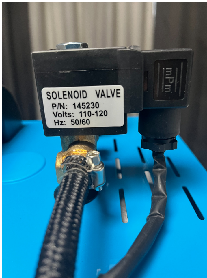
P/N 145230 steam solenoid installed in The Workshop Ledger ST-750 reference unit. The installed coil is marked 110-120 V and 50/60 Hz; the steam-hose connection and associated valve fitting are also visible.
