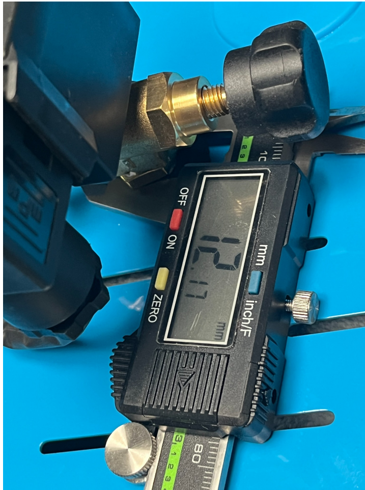
Digital caliper measuring the exposed threaded stem of the ST-750 steam-adjustment valve. The recorded outside diameter is 12.17 mm.
