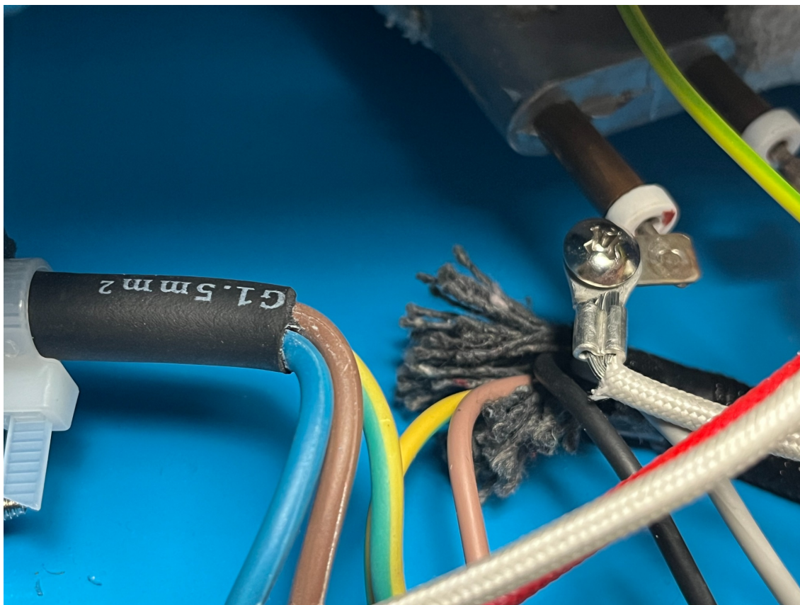
Frayed gray fibrous material documented within the ST-750 reference unit near the boiler and internal electrical wiring.
