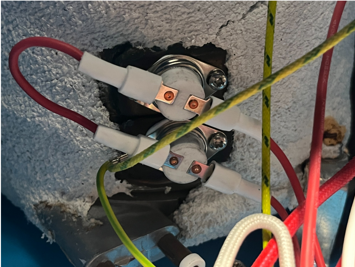
Two thermal devices mounted against the boiler of The Workshop Ledger ST-750 reference unit. Their individual switching functions and temperature ratings have not yet been established.
