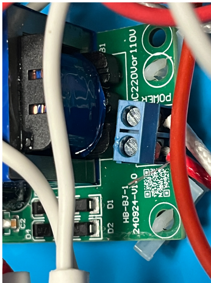
HB-BJ-1 electronic board, transformer and terminal end. The photograph documents the board identification, 240924-U10 marking, transformer, terminal connection, and associated wiring.
